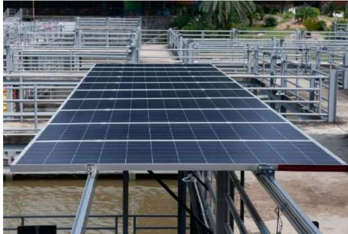
Figure 3: Solar Panels installed at Nong Nooch Gardens for the Big Thing
